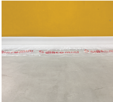
Laying of the wall insulation strip along the internal perimeter of the house.
